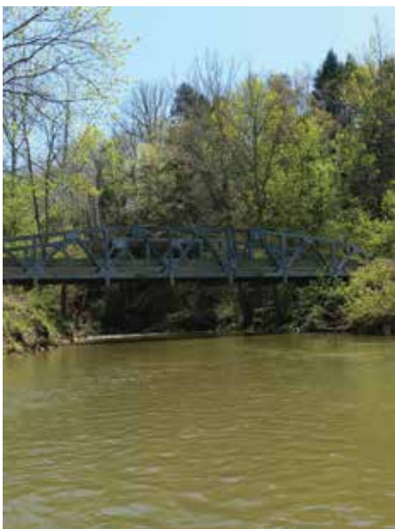
Tabbs Ford bridge. The only road crossing in the 13-mile stretch from routes 647 to 211, near the beginning of the journey.
